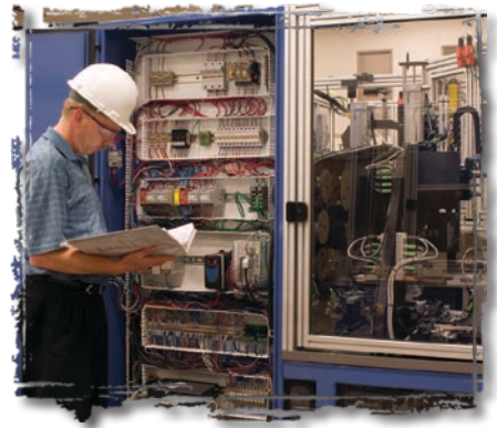
A Technologist examining an electrical control box.
