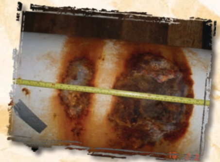
Corrosion on pipe. Courtesy of Spectrol Energy Services Inc.
